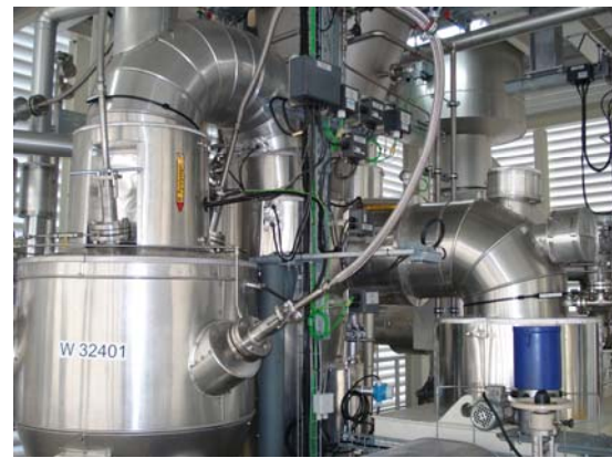
Figure 4: bioliq ® pilot facility [31,32]
